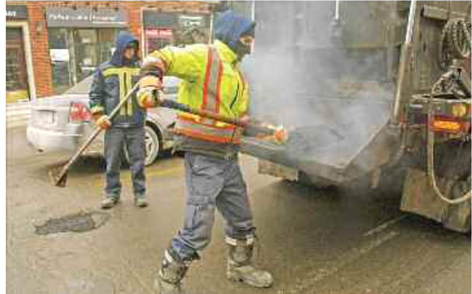
Public Works employee Marco Brunetti shovels hot, steaming asphalt from the back of a city truck as colleague Justin Cavanagh Jackson pounds it down into potholes on St. Catherine St. January 24. See story, p. 15.
