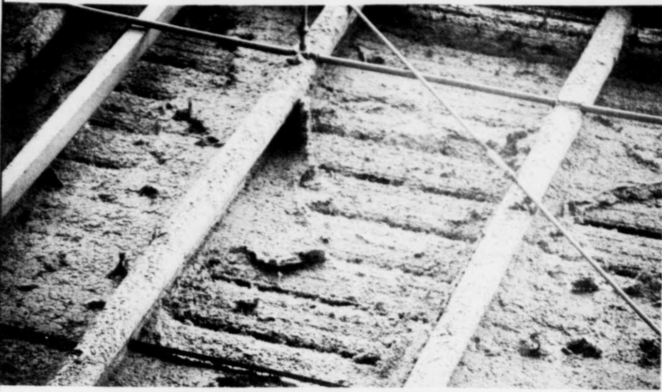
The ceiling of the Scott arena has been shedding its asbestosfibre insulation since it was sprayed on in 1961.
