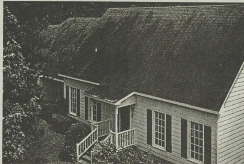
BLACK STREAKS caused by algae growth cover virtually the entire surface of this roof.
