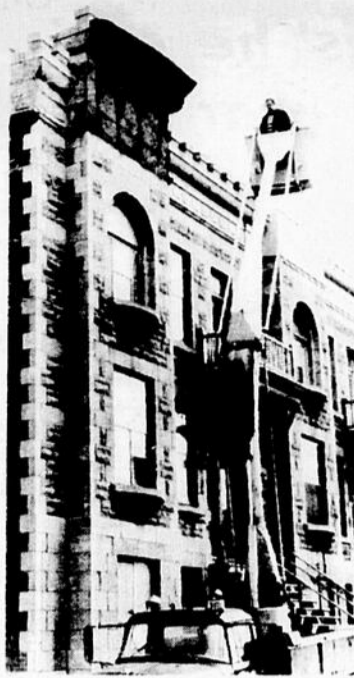
ROOFING FIRST AID: The city public works department's "cherry-picker" vehicle came in handy last Friday afternoon to patch up loose roofing tin flapping in the wind of this multiple dwelling at Blenheim place and St. Catherine street. Shortly before, a large sheet of the metal dropped into Blenheim in a spot normally occupied by a parked car.
