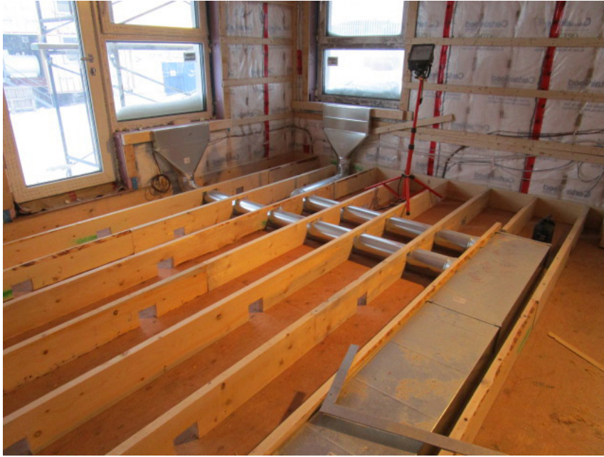
Figure 14: Ventilation ducts in the subfloor space
