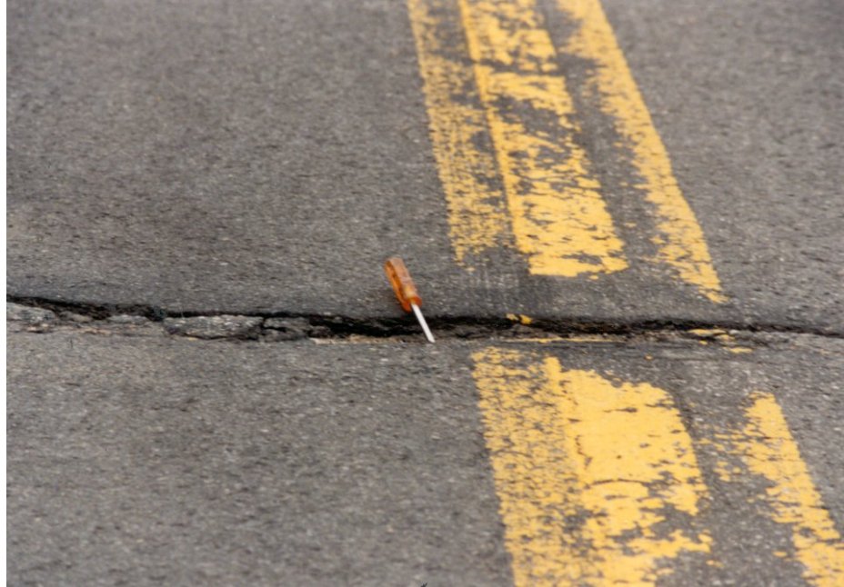
Photo 3.7.1 a) – Fissure transversale
