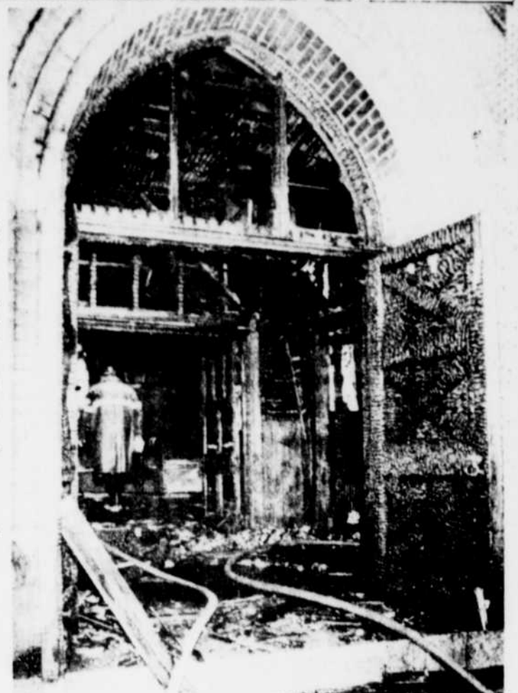
The QPF arson squad are investigating Tuesday's fire which caused more than $60,000 damage to St. George's Church in Granby.
