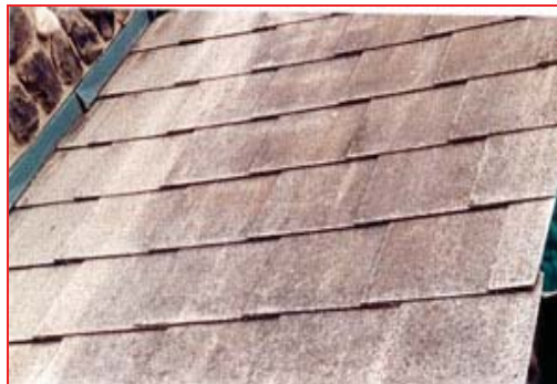
Asbestos material in roofing cc. Joseph Jenkins, Inc
