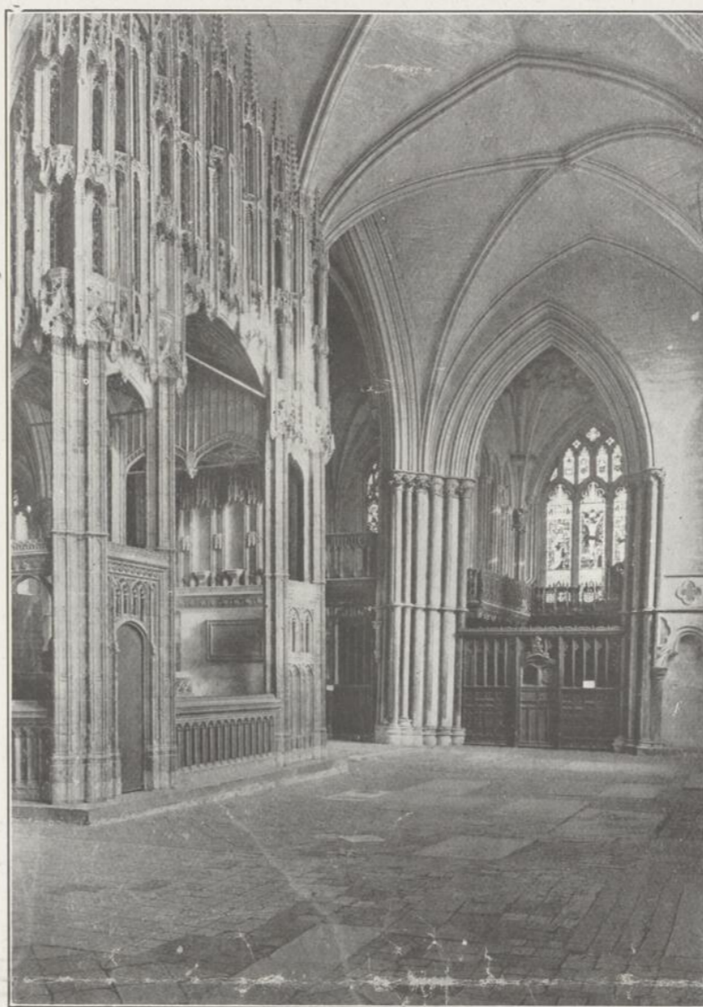
SAVING A CATHEDRAL FROM DESTRUCTION—The south transept of Winchester Cathedral, showing the extent to which it leans from the perpendicular owing to the sinking of the foundation. For six years now the work of renewing the foundation has been going on, with the result that the venerable building has been saved from what appeared to be imminent destruction. An exhaustive description of the manner in which the restoration was carried out, and the difficulties that accompanied the task, appeared in a recent issue of The Standard. (Photo by Arthur Hulme, Montreal.)
