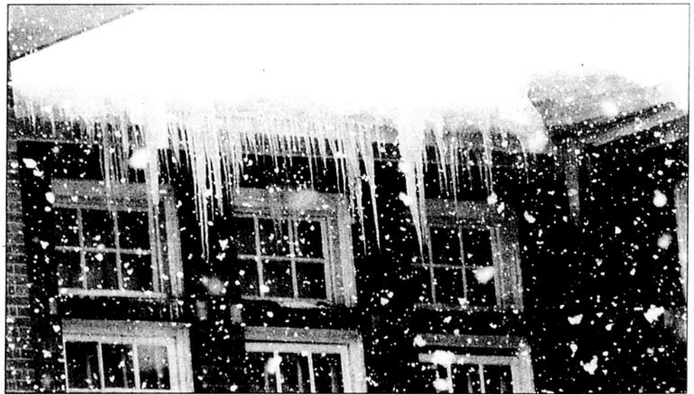
Large icicles hanging from the roof at Roslyn School have been removed since they forced part of the schoolyard to close for safety measures on March 12. (Photo: Martin C. Barry)
