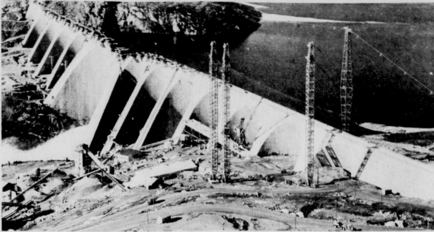
NEAR COMPLETION — Manic 5, largest multi-arch dam in the world, is the pride of Quebec engineers and construction crews involved in the seven-dam power development on the Manicouagan and Outardes rivers. The final ribbon of cement will be poured along its crown this spring. (CP Photo)
