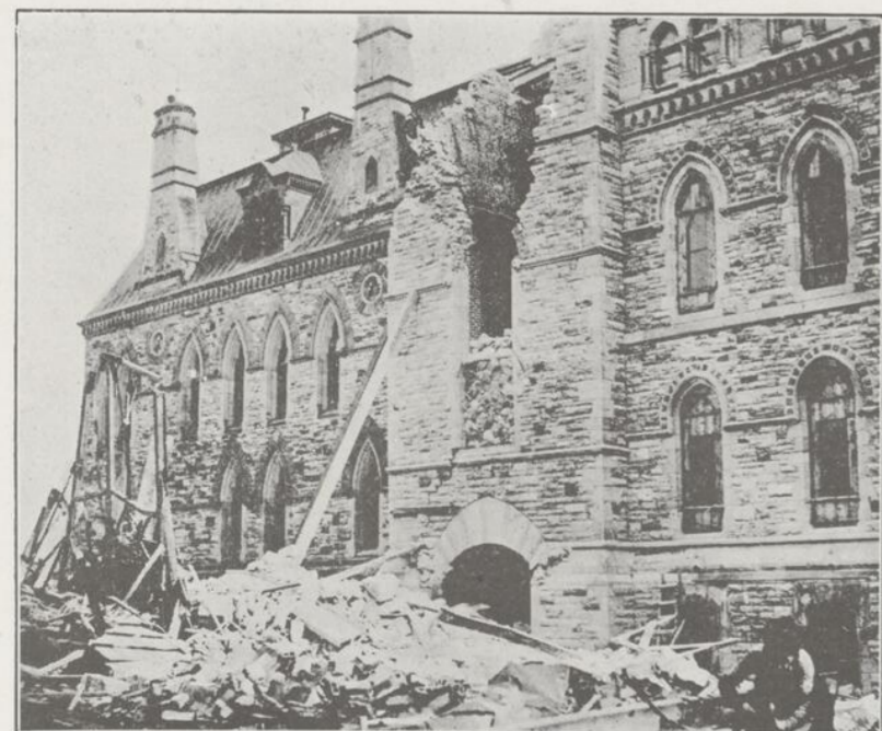
THE INVESTIGATION INTO THE COLLAPSE OF THE LAURIER TOWER AT OTTAWA—This tower, which was built during the past winter, recently toppled over, owing, it is said, to faulty construction. The Government is now making an inquiry into the cause of the mishap. It formed a prominent architectural feature of the Western Departmental Block.
