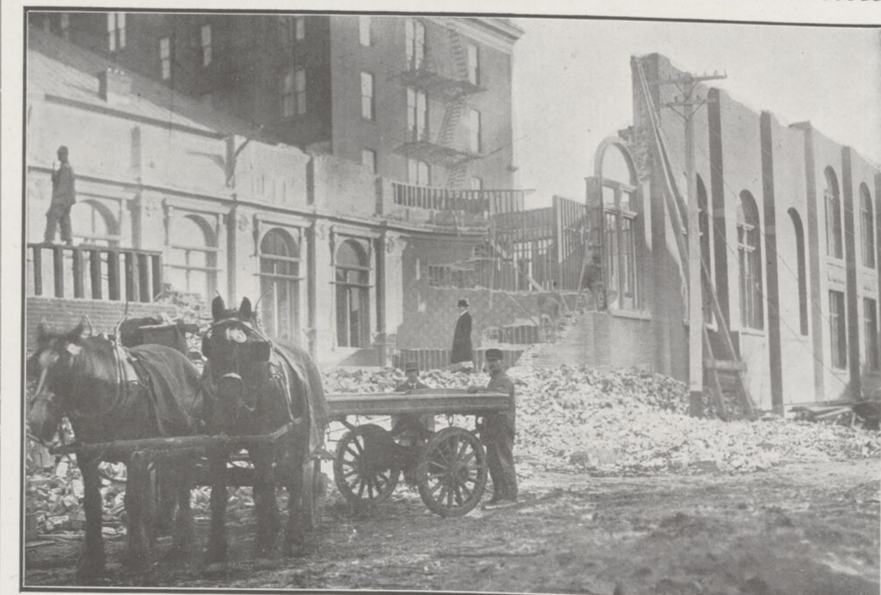
DEMOLITION OF THE WINDSOR HALL, MONTREAL—The work of razing this one-time popular concert hall goes on apace, and in a few days nothing will remain of the superstructure. In its place will rise a large and modern addition to the Windsor Hotel, which will greatly increase the accommodation of this hostelry.
