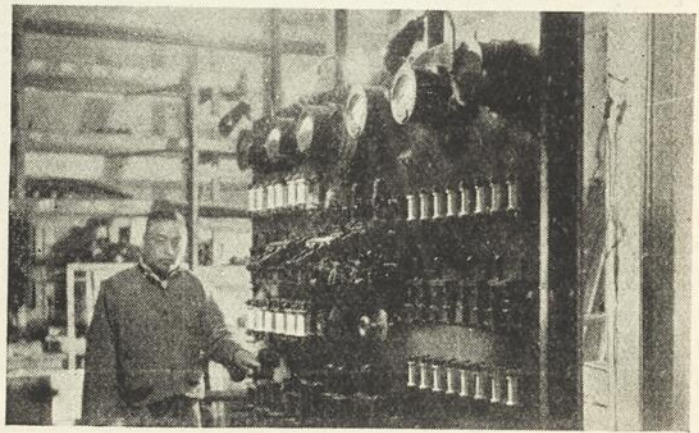
FIG. 2.—Main switchboard built by the new Engineering & Shipbuilding Co. Ltd., Shanghai.
