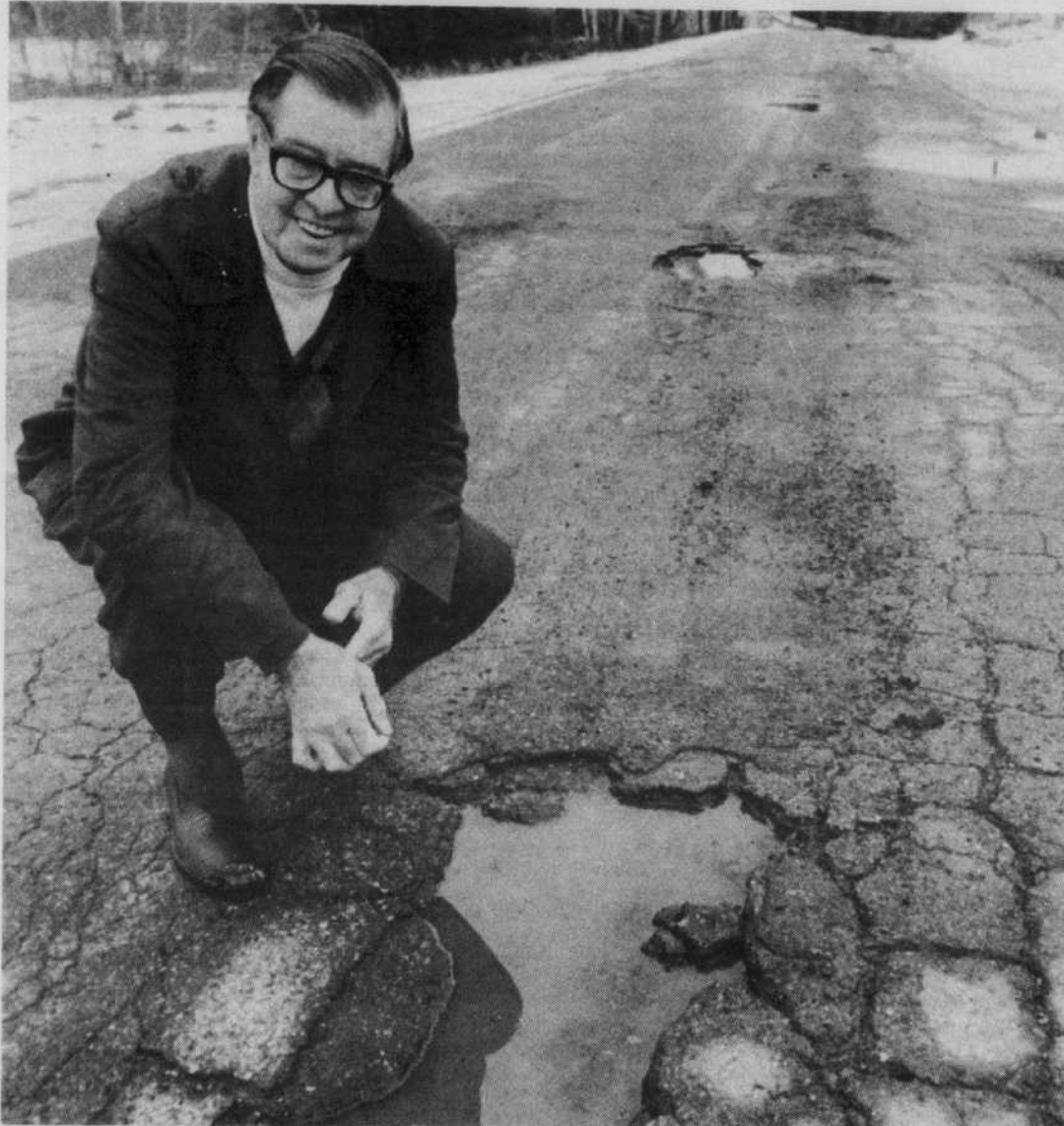
Reporter Gil Smith points to just one of the many potholes awaiting motorists on West Bolton roads.
