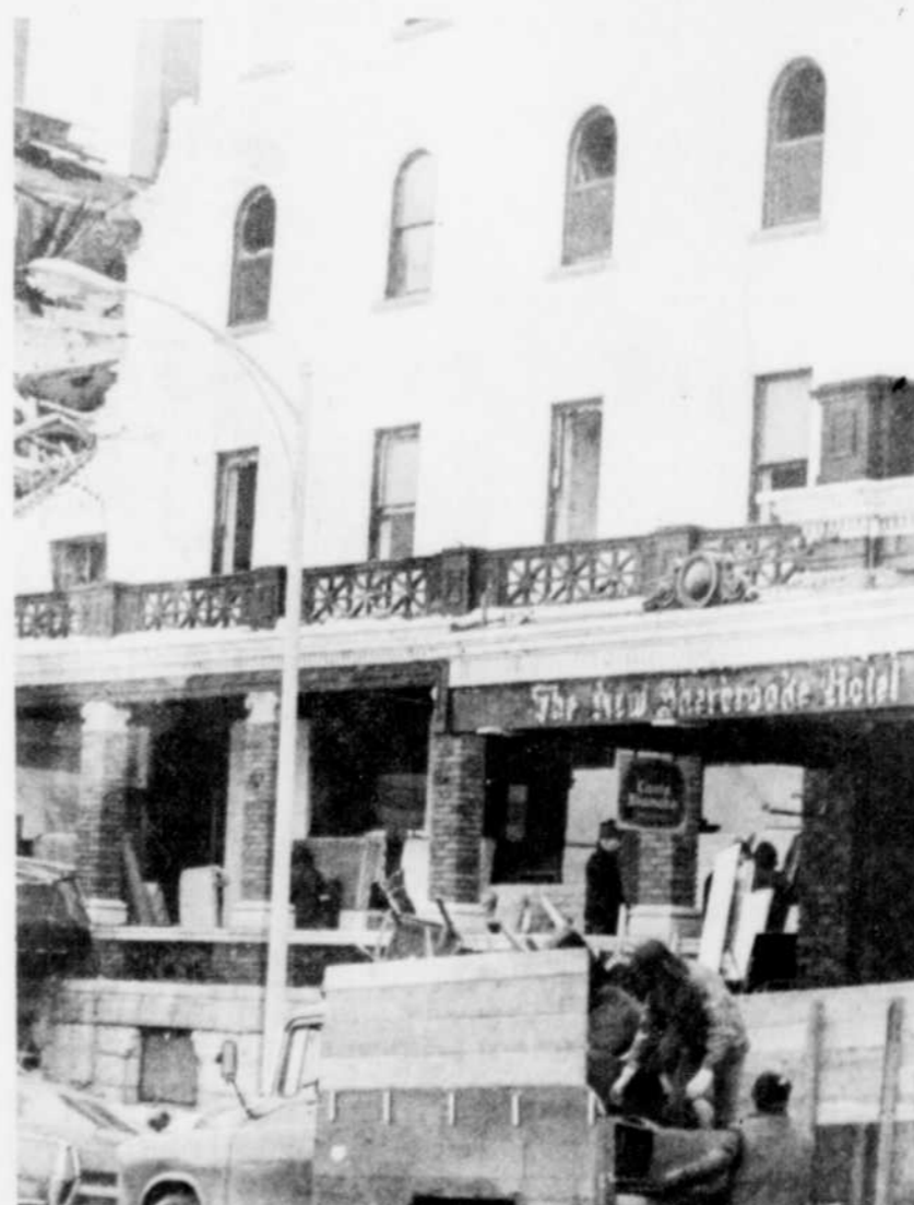
DEMOLITION STARTED — Work to demolish the ruins of the New Sherbrooke Hotel has started. Saturday a miniature auction was
