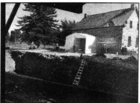
Excavating a wine cellar and and tasting boutique is part of the expansion project at the Hemmingford cider house La Face Cachée de la Pomme. (Photo: Phil Norton).
