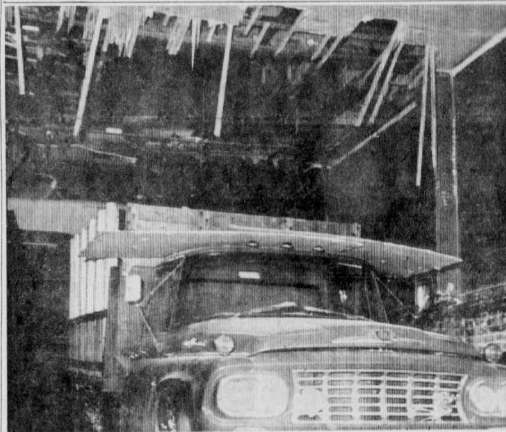
HOTEL DEMOLISHED — Demolition work started this week on the Windsor Hotel on Depot Street in order to make way for the city's Wellington Street South parking garage. The truck is shown here preparing to load up and cart off one of the ceilings in the building.
