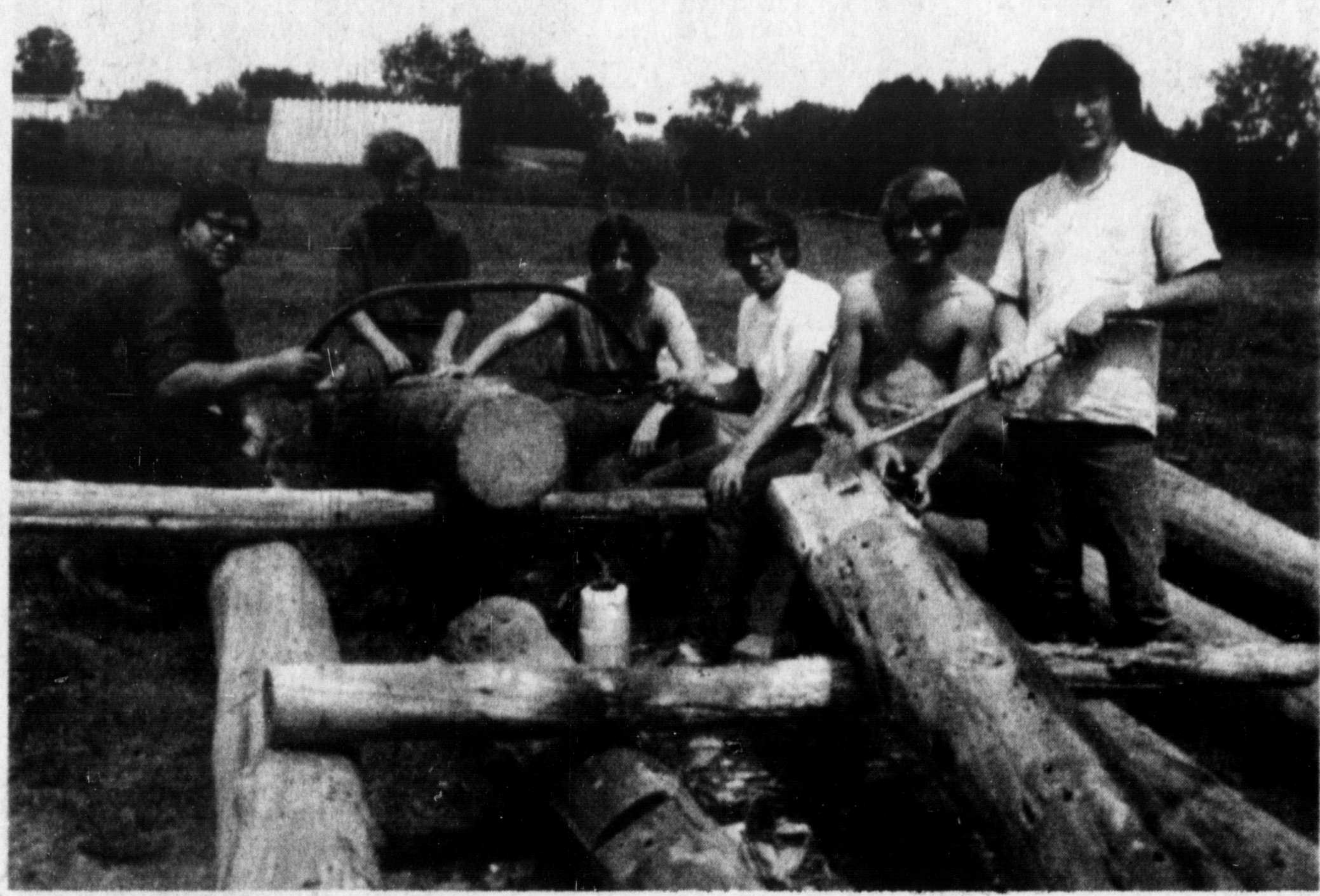
Building a bridge for the park in Shawville are Brent Bertrand, George Steeves, Steve Lydall, Ralph Bretzlaff, Terry Elliott and Colyn Steeves.
