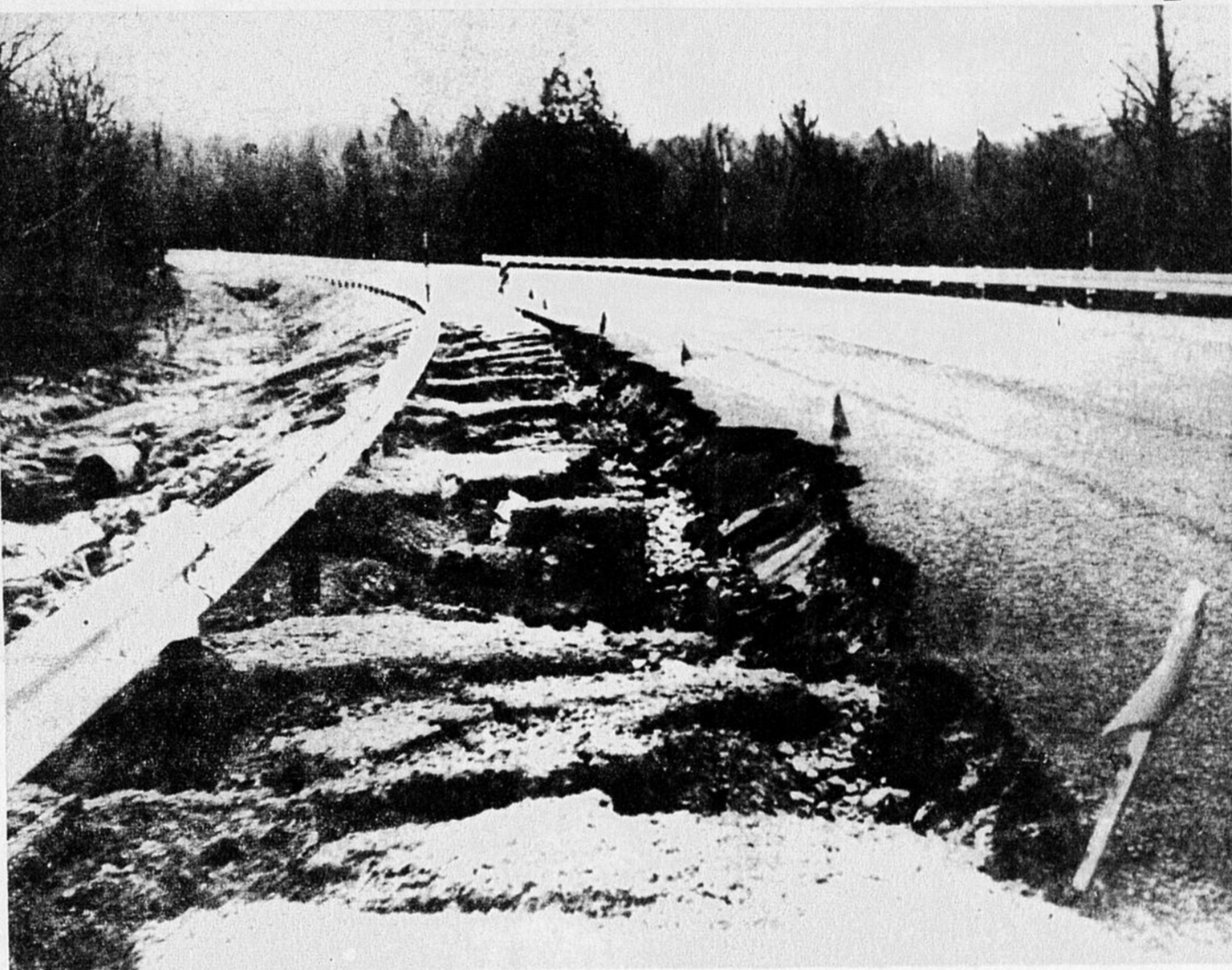
SPRING ROAD DAMAGE: April flooding in the spring run-off played havoc with the recently-constructed section of the Provincial Line Road between Herdman's Corner and the United States border. The freshet washed out the road
