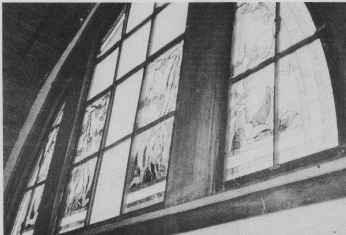
Maurice Biron and Ninette Sylvestre spent a year creating this unique stained glass window installed in the St. Elizabeth's Roman Catholic Church in North Hatley this summer.
