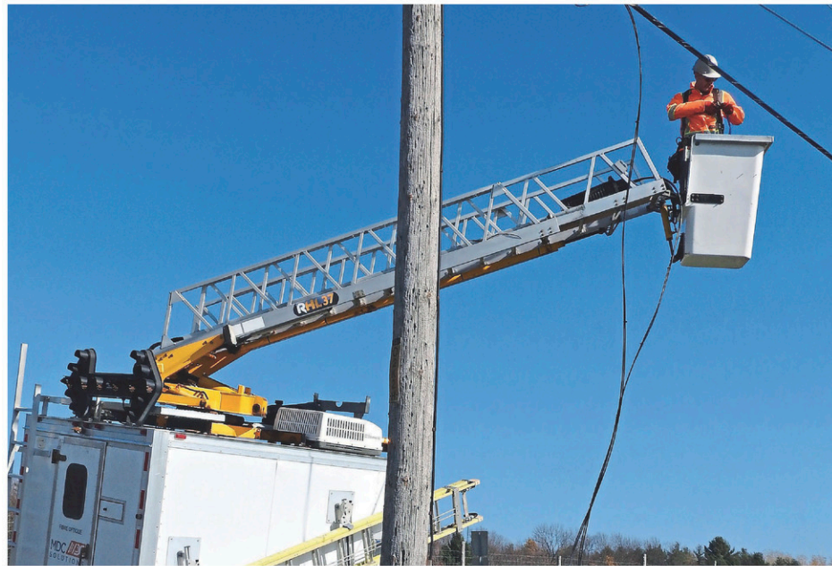
With the arrival of spring, cable installation will pick up speed as the weather makes it easier to repair poles and install cabling and equipment. (Photo: Courtesy)
