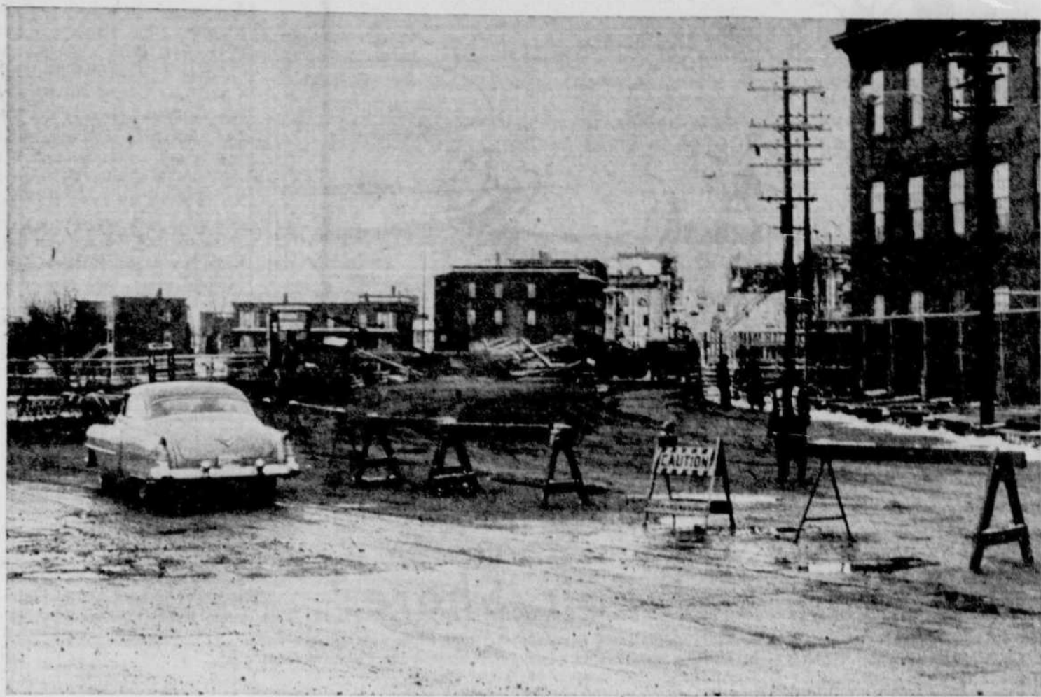
NEAR COMPLETION — While the new Montcalm bridge may not be opened by Thursday, the target date, the above photograph indicates the structure is nearing completion. Work on the bridge proper is finished and the preparation of the approaches has been considerably advanced. (Record Photo by Gerry Lemay)
