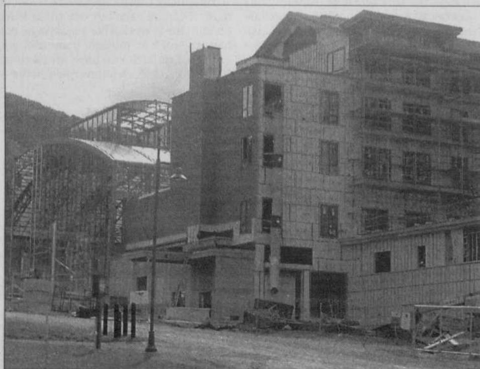
A view of the construction of Jay Peak's latest hotel with the attached indoor water park, which, along with the championship golf course, will help make the resort a four-season tourist destination in the Northeast Kingdom.
