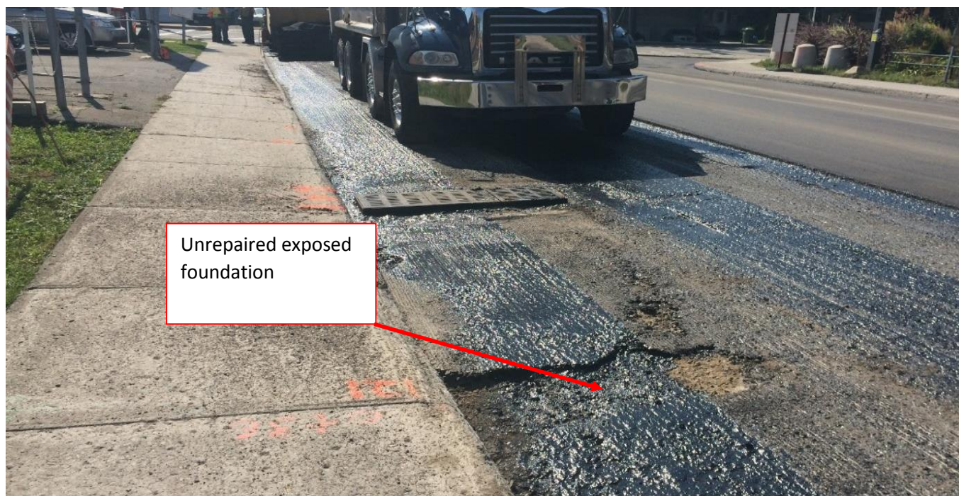
– Photo 1 taken by the OIG on September 17, 2015, on Monselet Street, illustrating an unrepaired defect that has reached the foundation.
