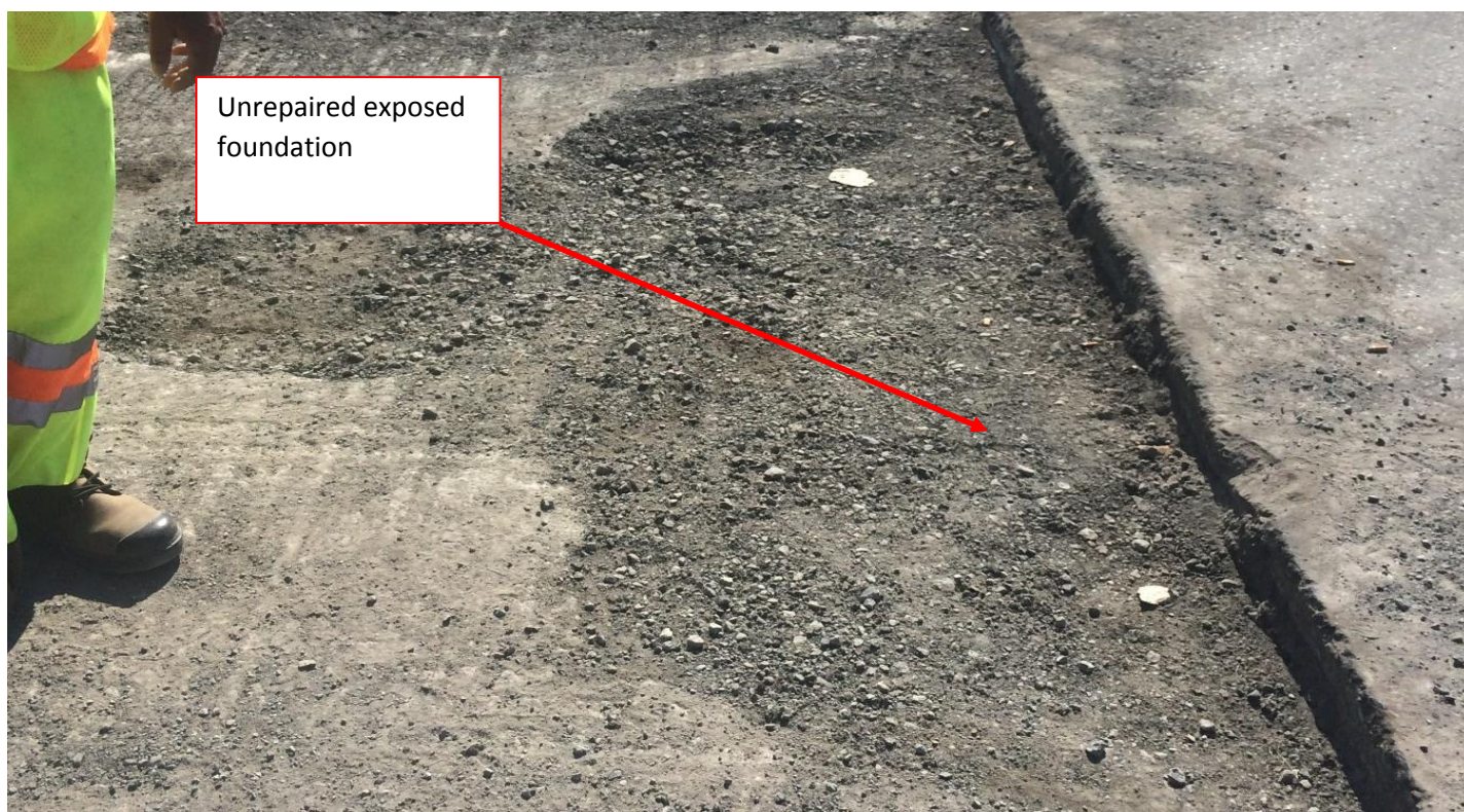
- Photo 6 taken by the OIG on September 17, 2015, on Monselet Street, illustrating an unrepaired defect that has reached the foundation.
