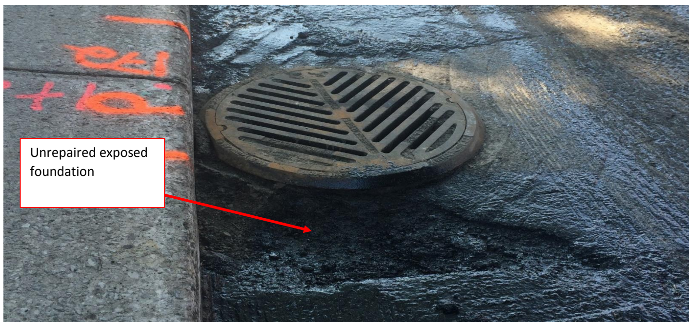
- Photo 5 taken by the OIG on September 17, 2015, on Monselet Street, illustrating an unrepaired defect that has reached the foundation.
