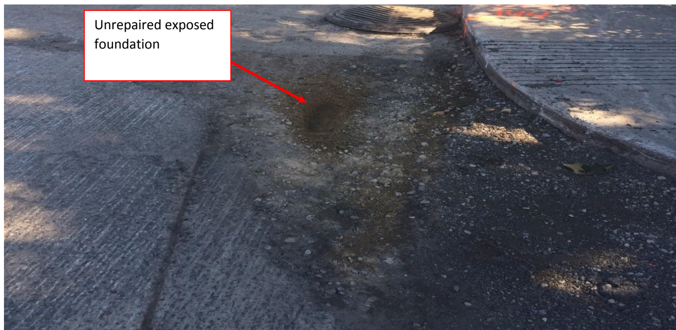
– Photo 3 taken by the OIG on September 17, 2015, on Monselet Street, illustrating an unrepaired defect that has reached the foundation.
