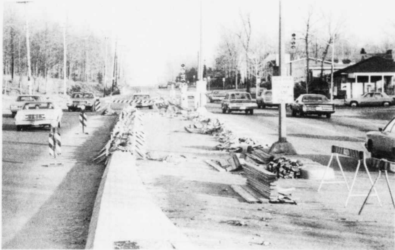
MUCH NEEDED REARRANGEMENT UNDERWAY — The intersection of Portland and Jacques Cartier boulevards is presently the site of some much needed reconstruction. When the work is completed, drivers will be able to take advantage of two
