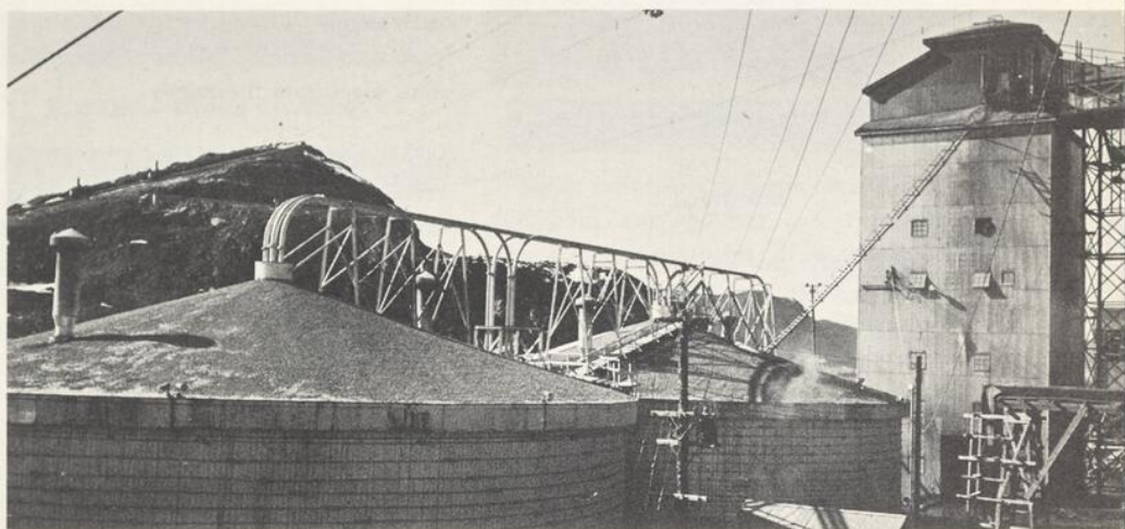
Two B.C. fir silos with interconnecting Fuller Kinyon lines are filled with cement. A Fuller Kinyon system reclaims the cement, delivering it to a batching plant in the background.
