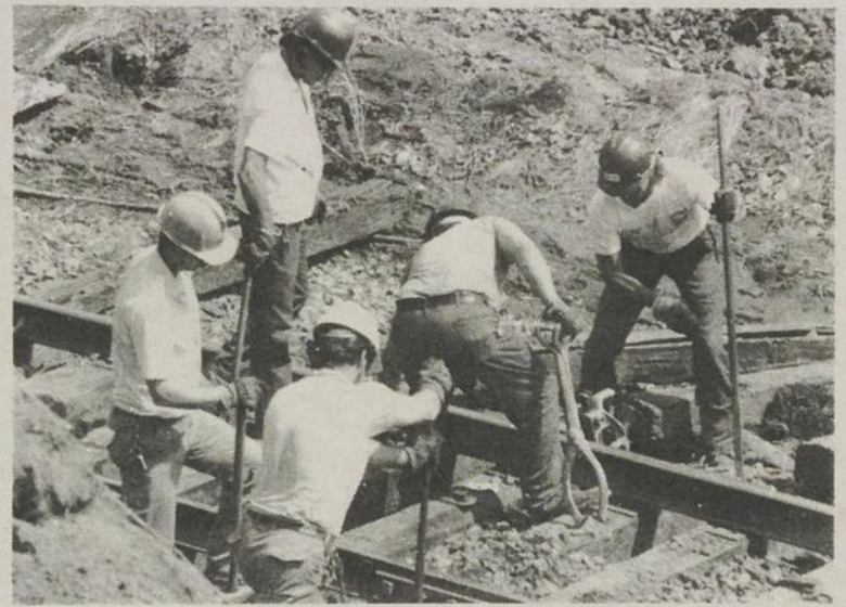
After the gas was gone repair crews started working around the clock to clean up and restore the tracks. They're still at it.
