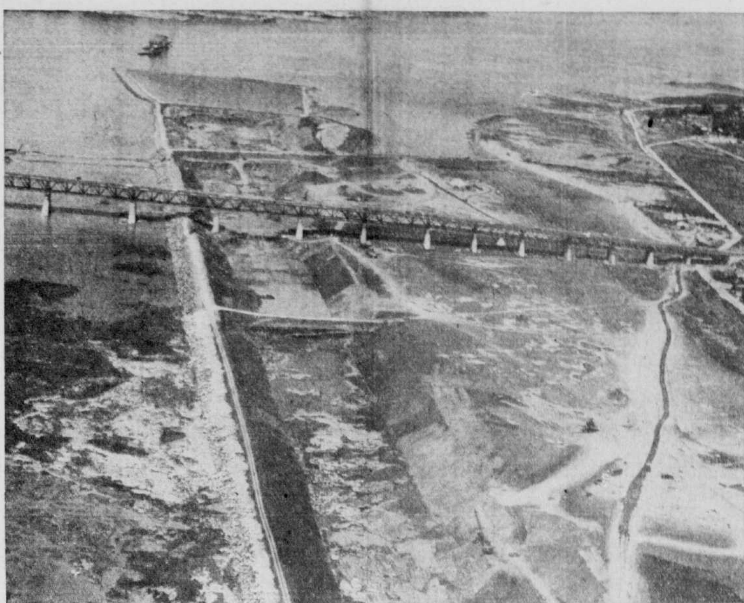
Seaway Progresses — Upper left is the future entrance to the St. Lawrence Seaway from Montreal Harbour. Vessels seen are dredges preparing channel entrance. Note good progress in excavation of Seaway Channel sloping rock cushion and outside high dyke to left. This portion of Jacques Cartier Bridge shown must be permanently elevated to provide 120-foot overhead clearance for ships using the St. Lawrence Seaway.
