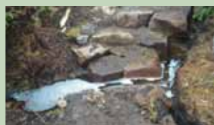
Rainbars that allow water to be evacuated outside the trail.
