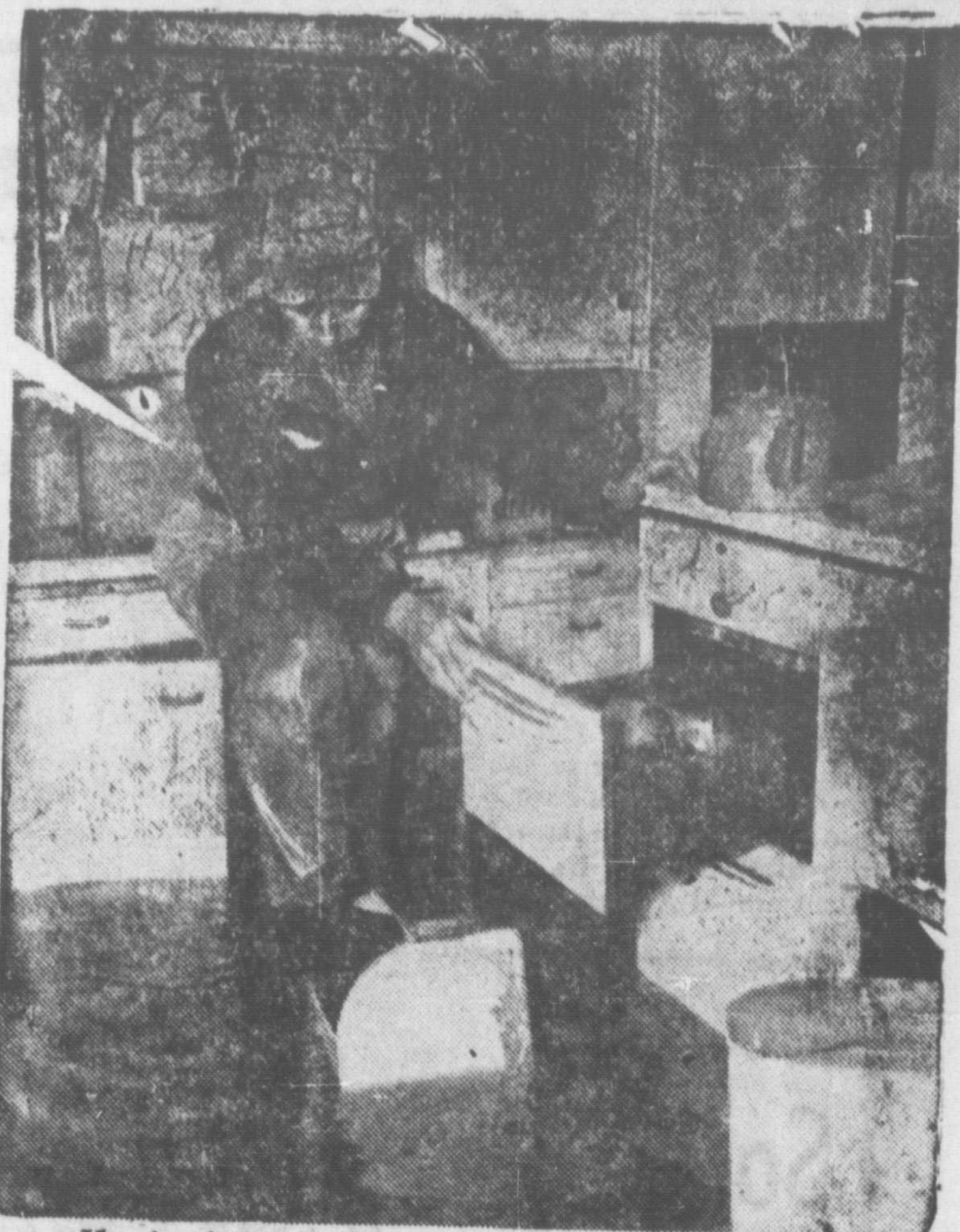
Here's what a kitchen in Morris, Manitoba, looked like after the Red River had done its worst. The warped cupboards, peeling paint, damaged kitchen utensils and almost unlimited quantities of mud and dirt, are illustrative of the damage done to F. Reeksiedler's entire home. Replacement of furniture, clothing, and personal effects is the responsibility of the Manitoba Flood Relief Fund. Contributions may be mailed directly to the Fund in Winnipeg, or paid into any bank in Canada.
