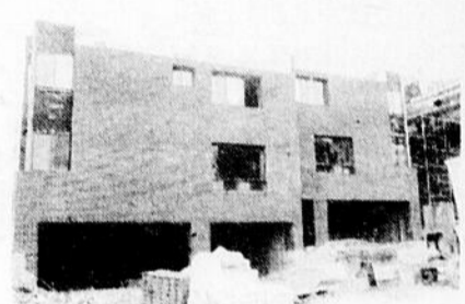
FOUR TOWNHOUSES UNDER CONSTRUCTION. Four bedrooms, den, two-car garage. Air conditioned. Wood floors. Fireplace. Skylight. Gourmet kitchen including eating area and laundry. $235,000 and $245,000. Edith Berman 934-1818; res. 935-4205.
