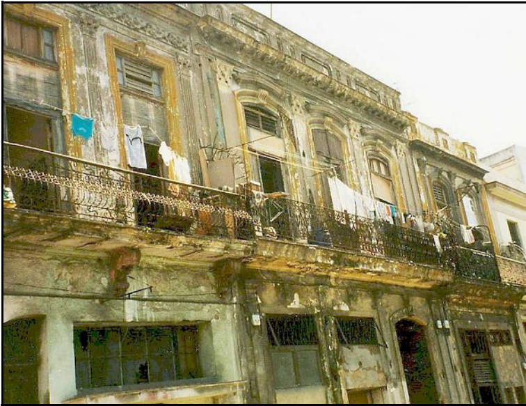
Figure 1.60: Buildings falling apart.
