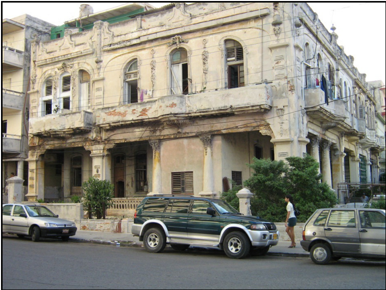
Figure 1.61: Typical photos near my hotel in Havana showing once elegant houses falling apart. Photo by F. Habashi.
