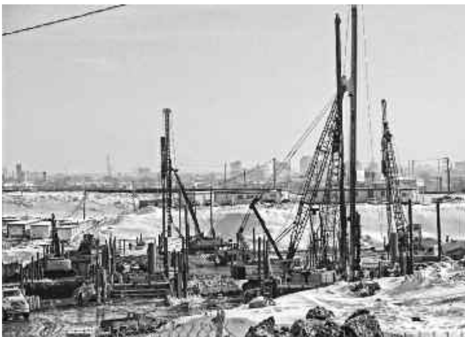
This was the scene on February 17 as piling activities continue at the incoming super hospital's Glen Yards site.
