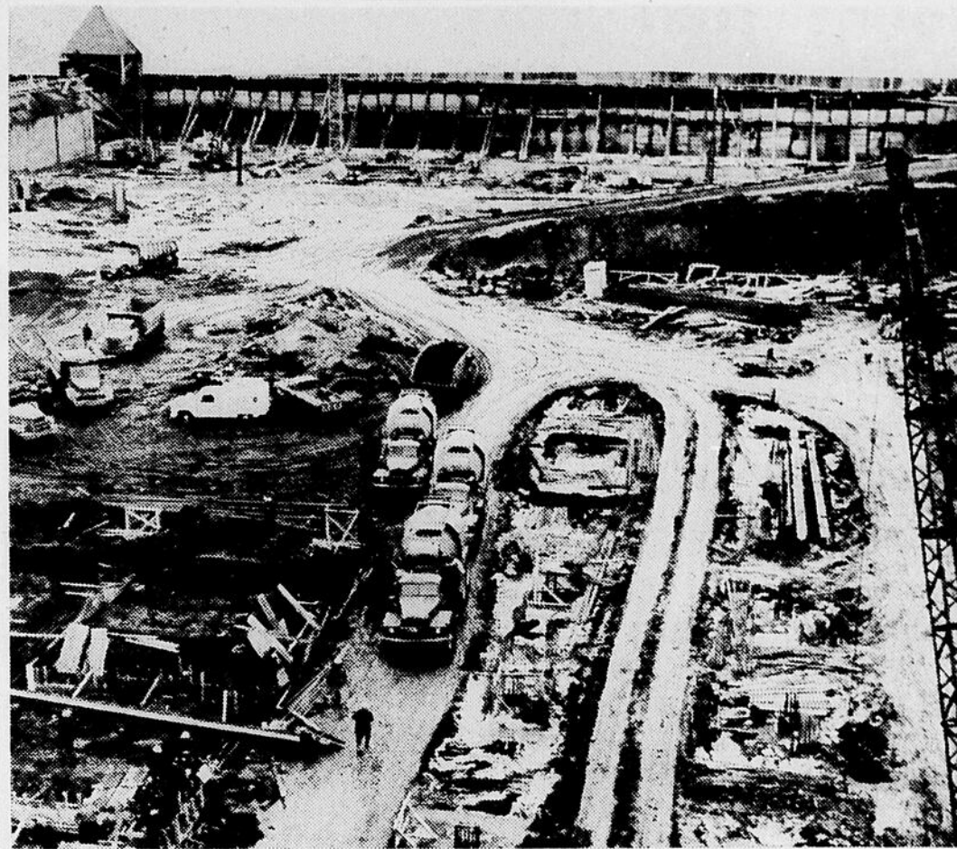
TAKING SHAPE: Work is beginning to take shape at The West End Plaza as workers battle cool weather and muddy conditions. In the upper left hand corner of the picture you can see where the steel work is beginning. Huge trucks are bringing in the steel every hour and each piece is labeled as to where it goes and how it fits. Elsewhere on the site, all concrete has been laid and most of the foundation work has been completed.
