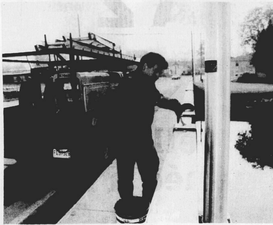
Since the removal of the old lamp posts on the Henderson Bridge there have been six potentially dangerous gaps in the railing. Workers originally roped them off where hundreds of Arthur Pigeon High School students pass daily. Now the gaps have been filled. Welder Jean Lavigne from the company Soudure et Location AFC in Ville Lemoyne completed the work on Tuesday, June 2.
