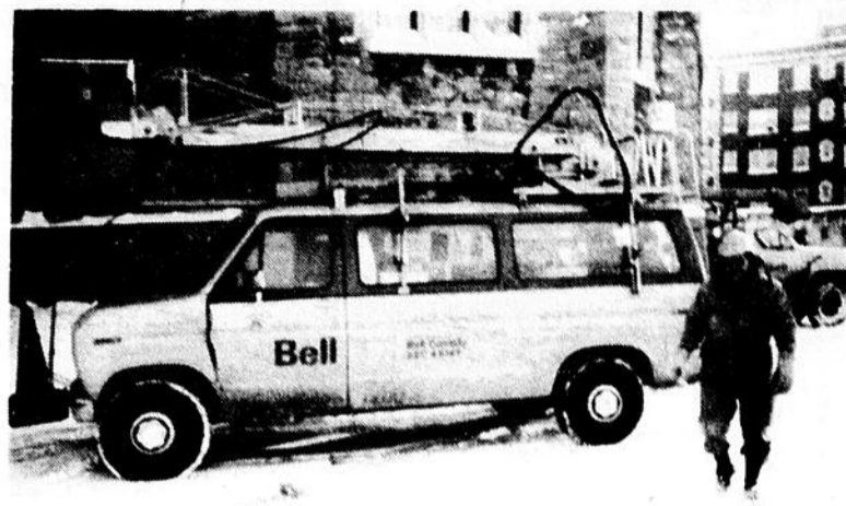
MA BELL TAKES OVER: Installation of the new phone system for city hall moved into high gear Monday with the rewiring of telephone equipment and installation of the computerized switch, the core of the SLIMS system. It is expected to be in operation by Jan 20, increasing the number of extensions from 90 to 120. Basic cost of the installation is about $31,000, with other costs to be amortized over a seven-year period.
