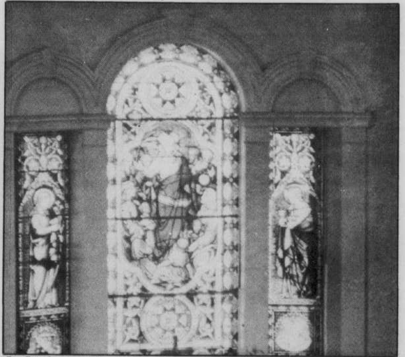
St. Stephen's stained glass windows are badly in need of repair.
