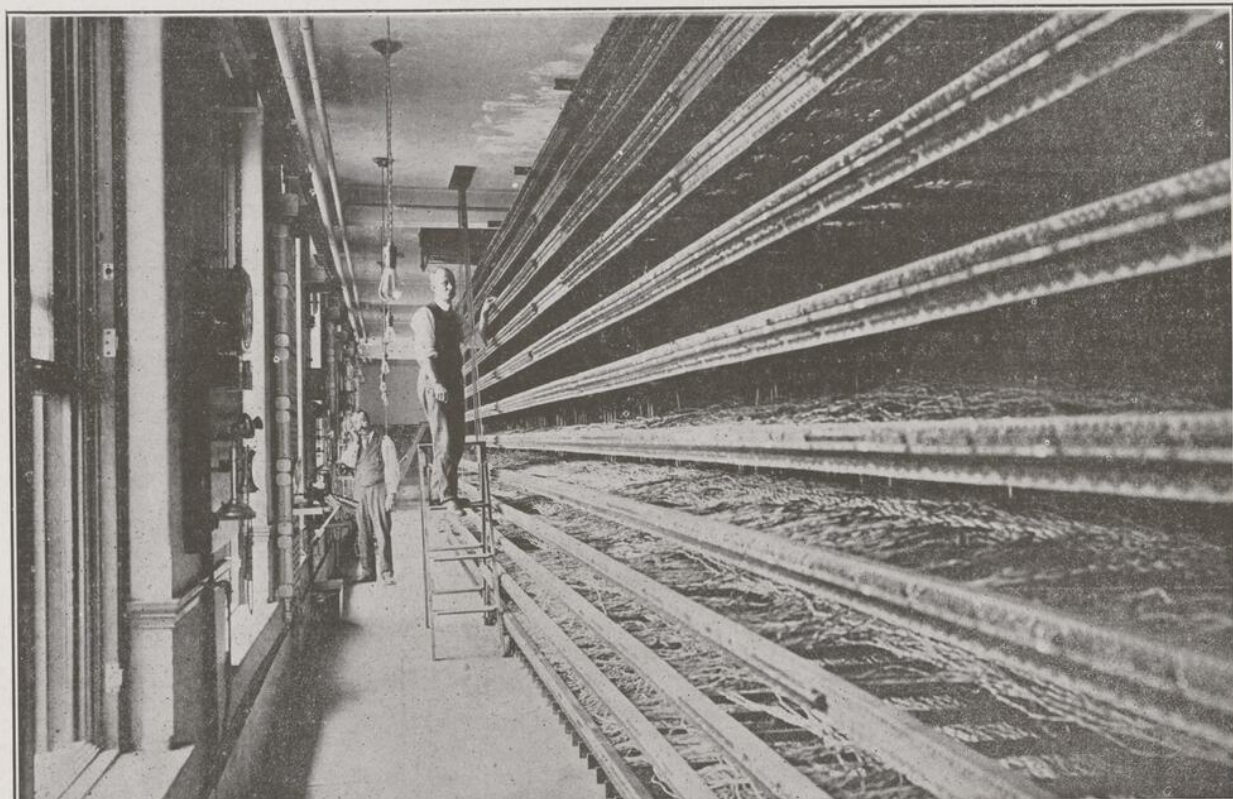
FIRE SILENCES THE 'PHONES OF MONTREAL.—At the Main Exchange of the Bell Telephone Company in Canada's commercial metropolis, three shifts of men have been at work for nearly two weeks repairing the damage wrought by a recent fire. This fire had the effect of silencing all the 'phones on this Exchange and temporarily cutting off communication over the long distance wires. To repair the damage, 50,000 wires will have to be spliced and 190,000 solderings will have to be made. It will be two weeks yet before the service is in running order again. The above picture shows the back of "A" board, and the racks of cables that were destroyed.
