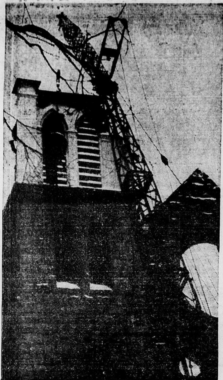
Lecompte & Fils working for the city of Valleyfield last Tuesday started with the demolition of the remains of the St. Mark's Anglican Church in Valleyfield. Here the large crain can be seen in action lifting the bell from the belfree. (Sun-Photo)
