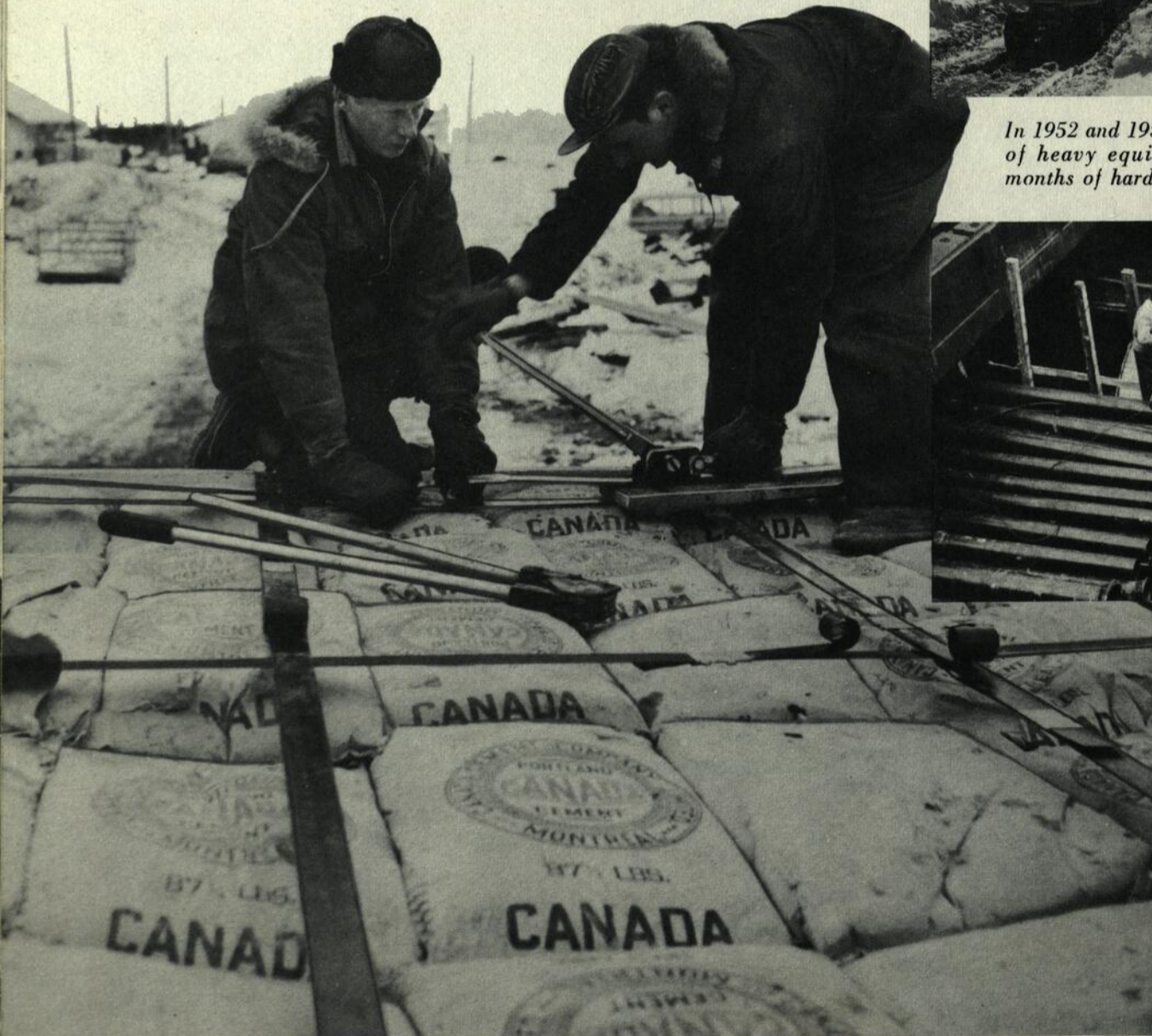
Some of the 190 thousand bags of cement used to build Menihék dam and power plant are loaded for shipment to the head of rail; from there they will be airlifted to the site of construction.
