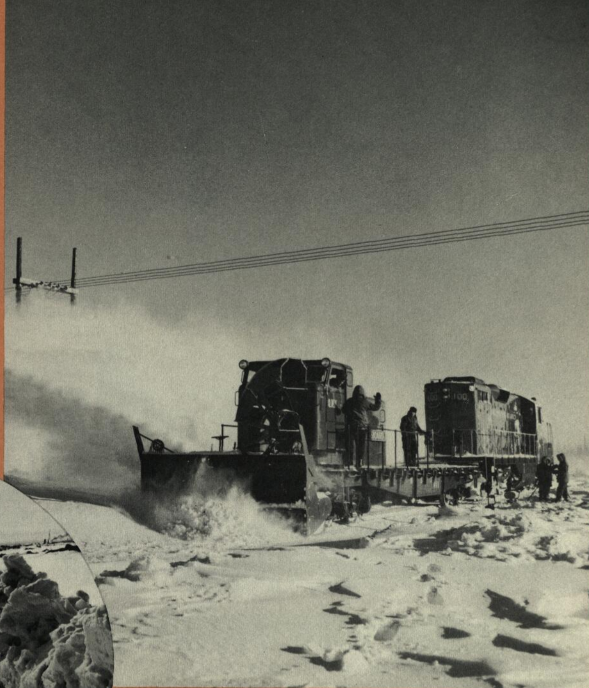
Modern snow-fighting equipment was used against storms severe enough to interfere with winter construction. Rails would drift over in a few minutes (below).
