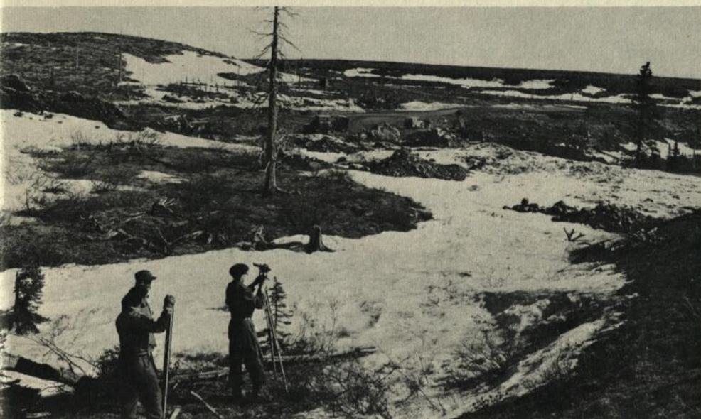
A survey crew marks the line a railroad spur will take past Burnt Creek to the Gagnon deposits and other ore bodies to the north.
