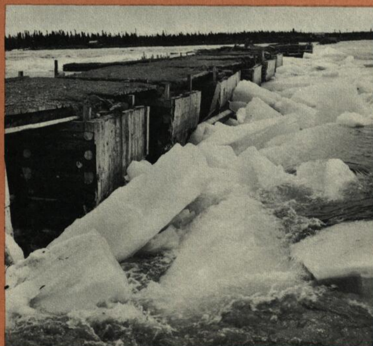
There was a sudden ice break-up and exceptionally heavy run-off in the spring of 1952 at the Menihok power project. Huge ice rafts swept down on the cofferdam bridge, causing extensive damage. Peak flow was estimated at 71 thousand cubic feet per second.
