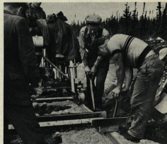
Ballasting, track raising, and tamping complete the operation. Mechanical ballaster tamps a tie in 7-8 seconds.
