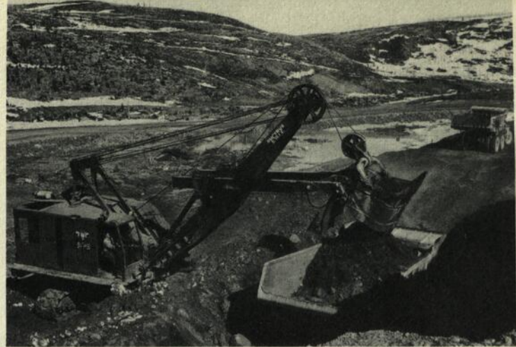
Shovel loads ore into a waiting truck; some of the first ore shipped will come from here.
