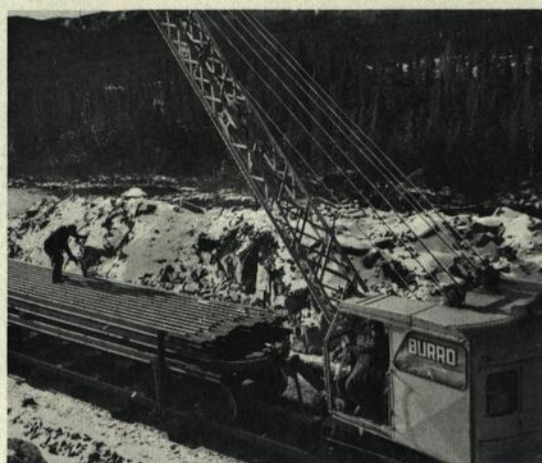
At the head of rail, a crane lifted off individual 132-pound rails as they were needed.
