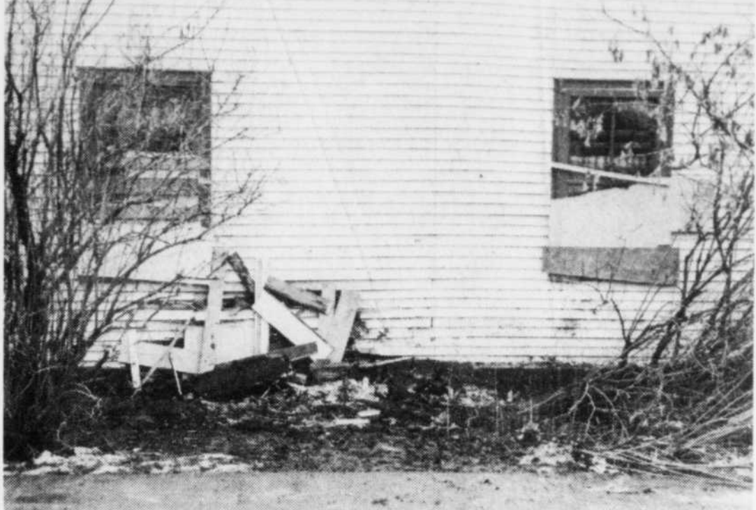
BUILDING DAMAGED — The wall of a building at the corner of King East and Curtis Street was extensively damaged early Sunday morning when a car went out of control and struck the side of the building. Although Sherbrooke Police refused to release information about the accident pending completion of their investigation, the Record has learned that one occupant of the car was killed and the passenger was taken to hospital. (Record photo by James Bruce)
