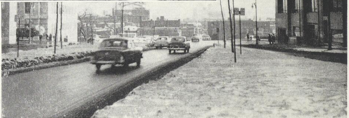
Digging foundations of Queen Elizabeth Hotel which is to stand beside Central Station, Airlines Building, Sun Life Building and St. James Basilica. — Alongside the Airlines Building, University Street has been opened below Dorchester, providing a new wider and split lane way downtown.
