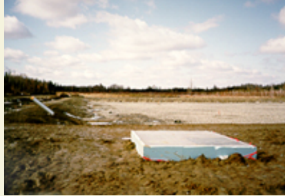
An experimental biological filter has been installed at the outlet to treat contaminated drainage water.
