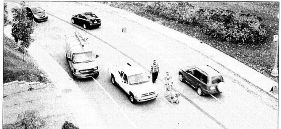
Residents of 200 Lansdowne say the new bike path in front of their building, seen here under construction in late October, presents a serious hazard. Photo: David Asch
