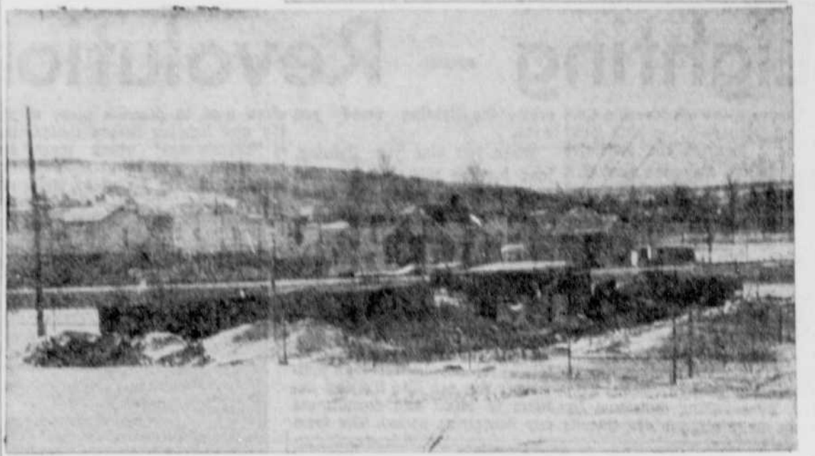
Foundation for the City of Magog's new electrical substation rises in the city's east section. (Record Photo by C. Catchpaugh)
