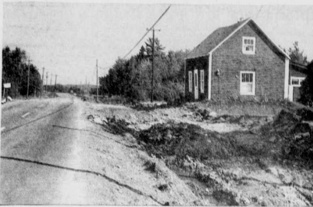
TOO CLOSE FOR COMFORT — This house on the St. Elie road, like five others on the two-mile stretch under construction, will have to be moved back because it is too close to the proposed road. (Record photo by Gerry Lemay)
