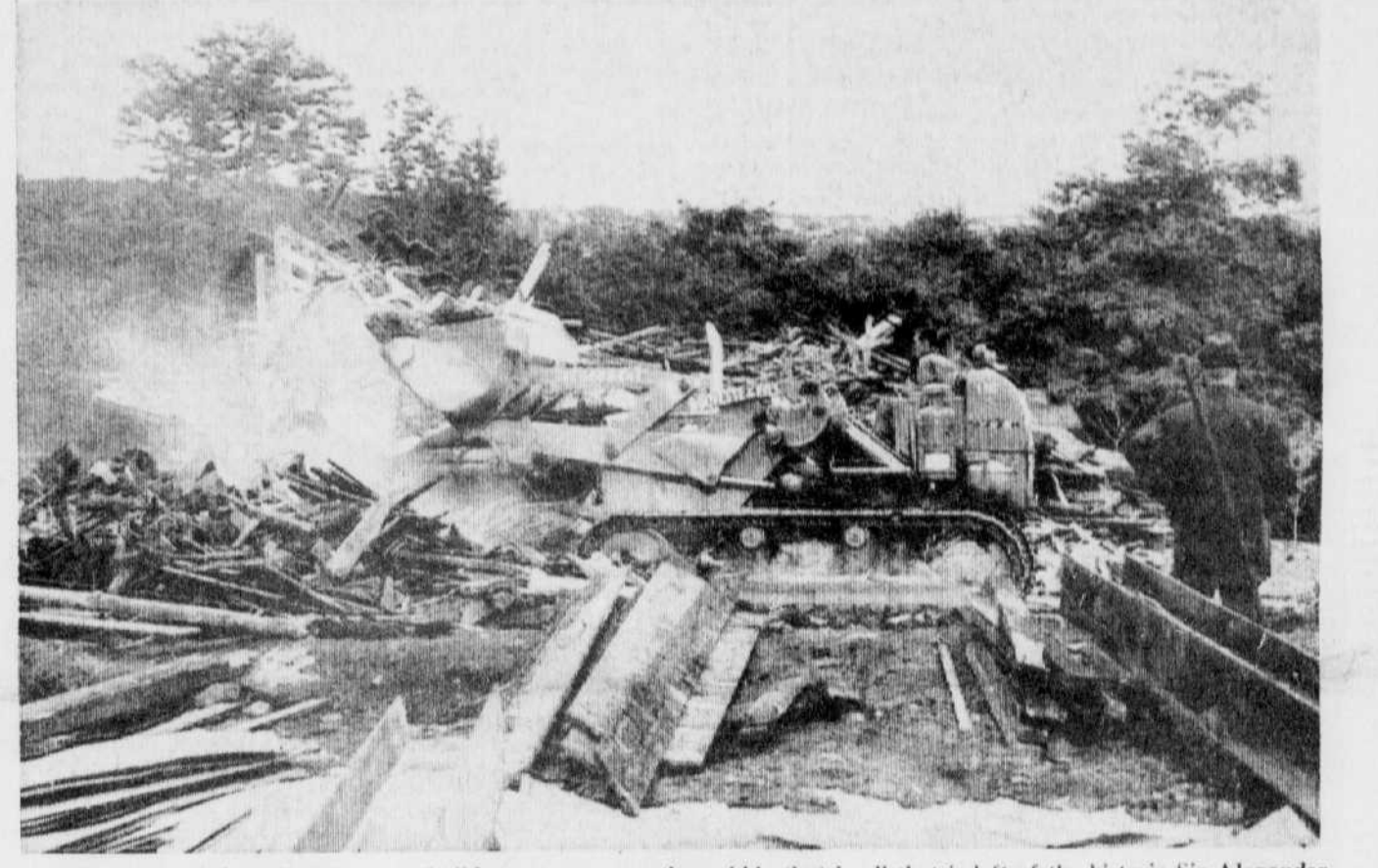
HISTORY BULLDOZED — A bulldozer scoops up the rubble that is all that is left of the historic Sir Alexander Galt home. (Record photo by Gerry Lemay)
