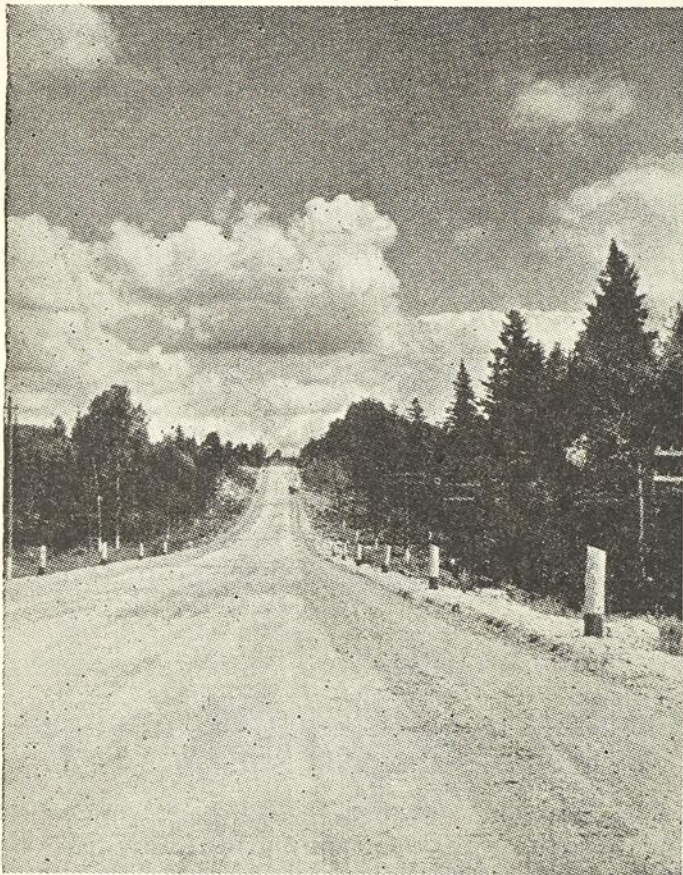
The finished road base, stabilized with common salt, will provide a strong and enduring foundation for the asphalt highway.
