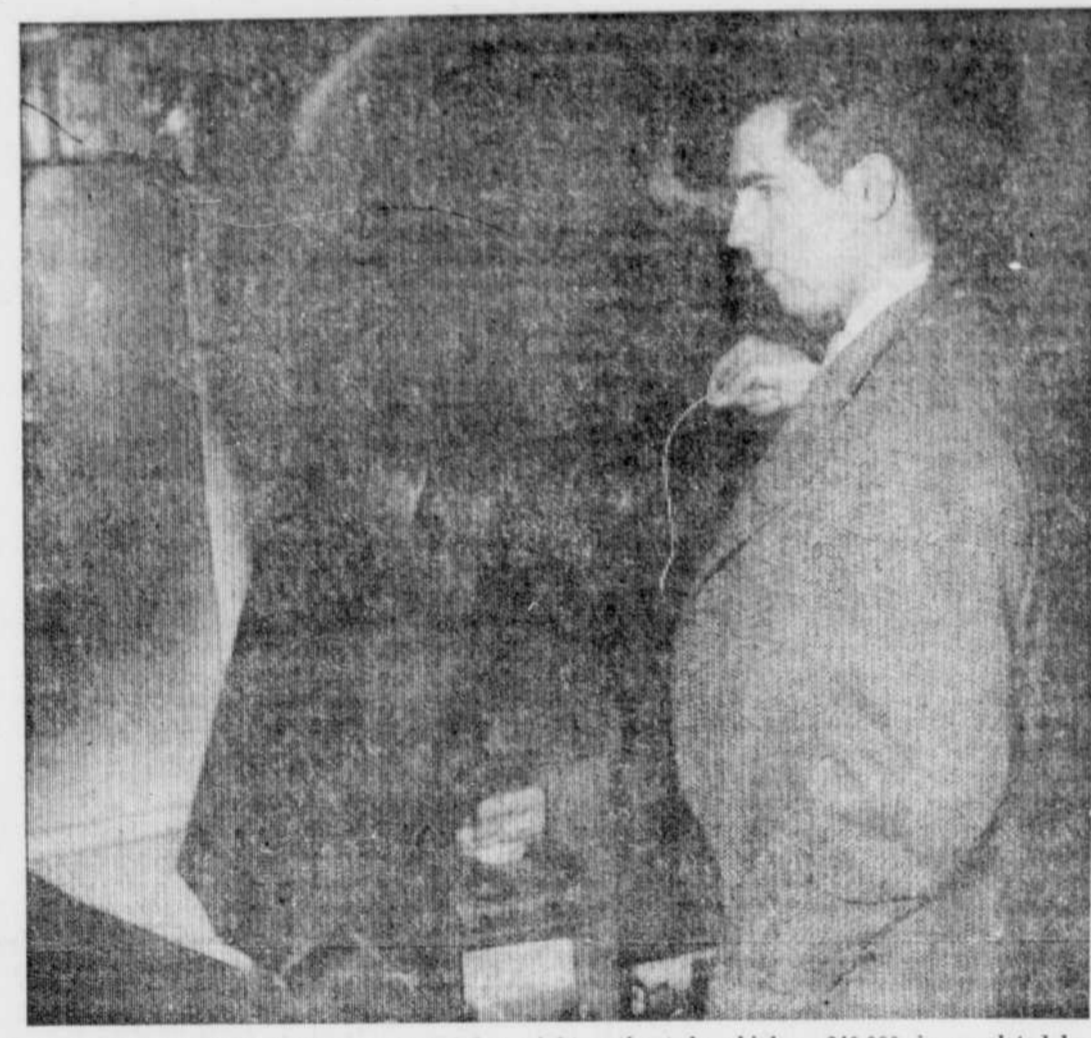
INSPECTION OF FIRE DAMAGE caused last night, estimated as high as $40,000, is completed by L. Dussault, of East Angus, co-proprietor of Ben's Bar-B-Q restaurant on Main street. Damage to the wall caused by burning cooking grease may be seen at the top of the picture. The restaurant is considered a complete loss. The fire broke out late last night in the kitchen of the basement restaurant. See story on page three. (Record Photo by Gerry Lemay)
