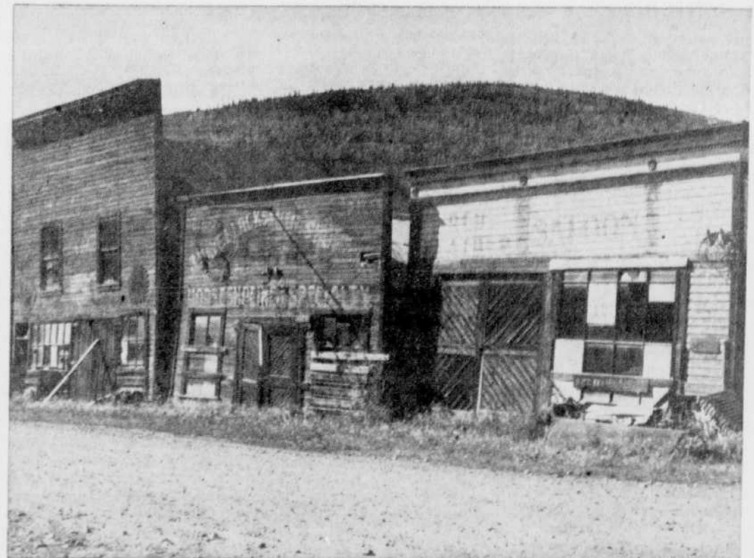
Abandoned and twisted by permafrost, old buildings such as these are numerous. (CP Photo)
