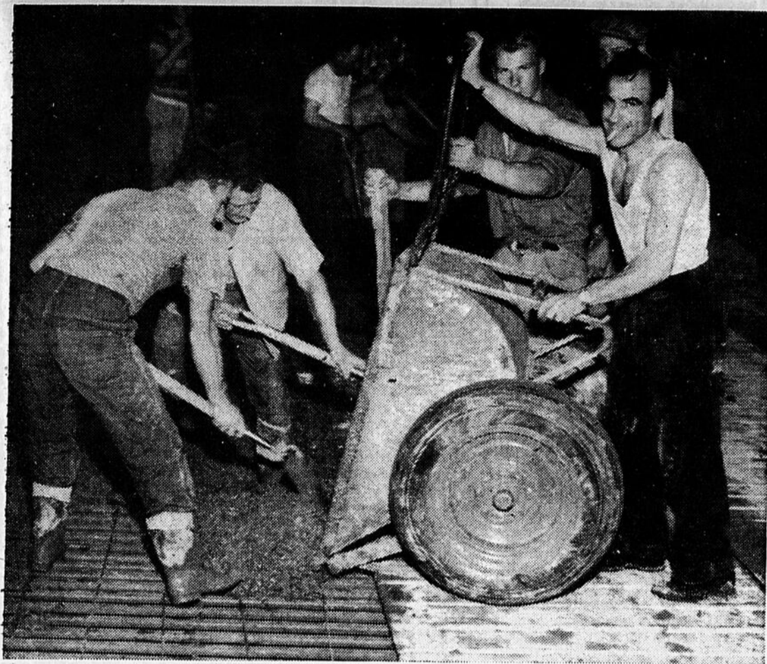
Workmen pictured at the recent pouring of the concrete slab at the artificial ice rink. This operation marked the final major portion of construction at the $580,000.00 structure which is now ready for use and will be opened early in the fall. Started on September 27th, 1957, the rink boasts the largest ice surface in Canada and excellent facilities for skaters and hockey players. There are six dressing rooms, four of them for hockey teams, which can accommodate 300 persons at one time. The slab was poured in a continuous 24 hour operation to prevent any seams in the concrete.
