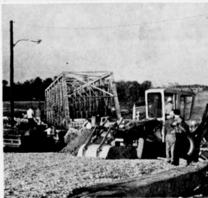
LIFT AND DROP — The Bromptonville bridge was closed to traffic yesterday evening, while engineers performed the arduous task of lifting the bridge and moving it over onto temporary foundations. A new bridge will be built on its former location.
